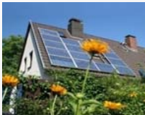
Solar Power Inverters
